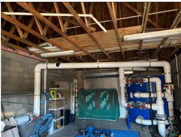
Figure 51 Pool mechanical room
