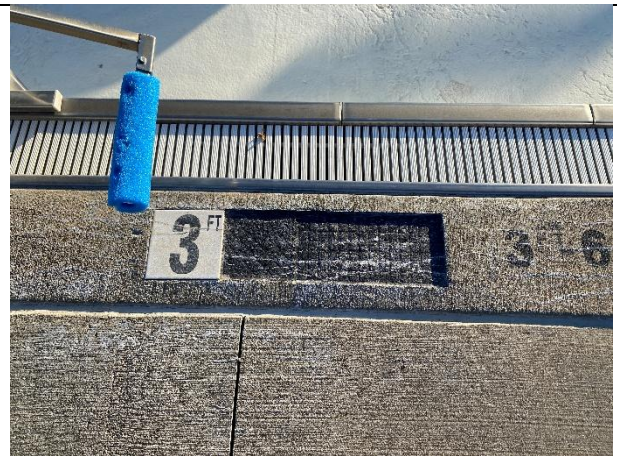
Figure 36 Missing depth markers in 3'6" area
