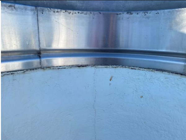
Figure 21 Vertical wall cracking in pool corner
