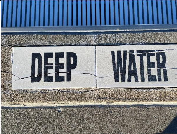
Figure 31 Cracking through deck edge and deep water markings
