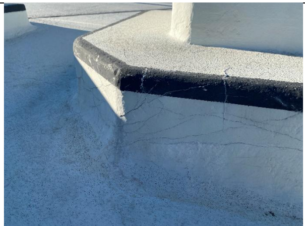
Figure 12 Cracking on underwater seating bench
