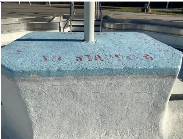
Figure 11 Cracking on therapy pool island
