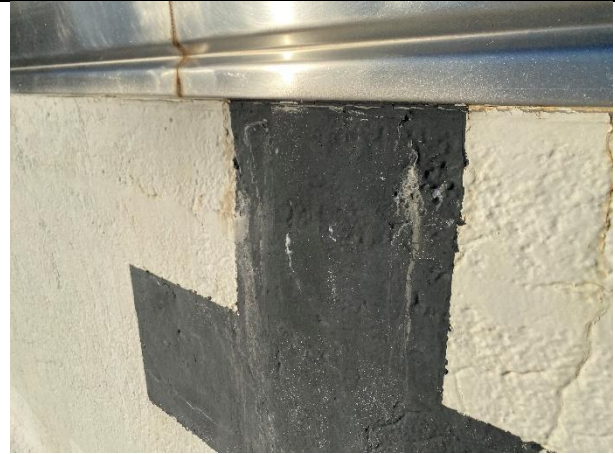
Figure 20 Concrete pitting around pool wall lane target
