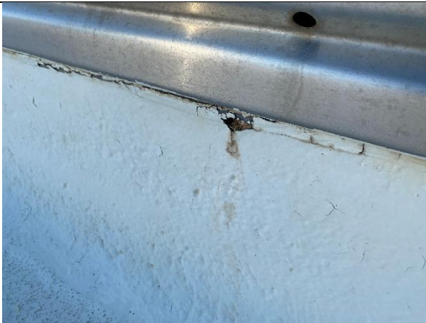
Figure 15 Concrete chipping under pool gutter
