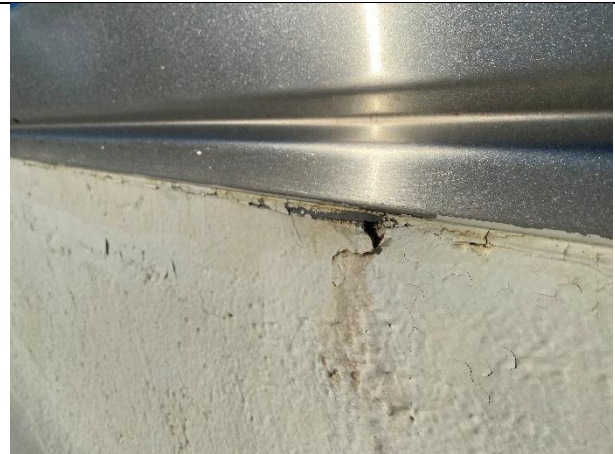
Figure 16 Exposed concrete under pool gutter
