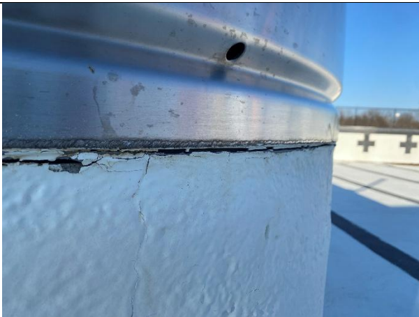
Figure 17 Gaps between pool wall and gutter
