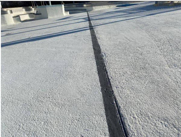
Figure 23 Swimming pool expansion joint
