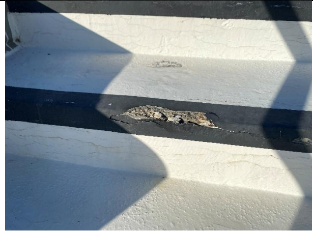
Figure 14 Concrete failure and delamination in pool stair entry
