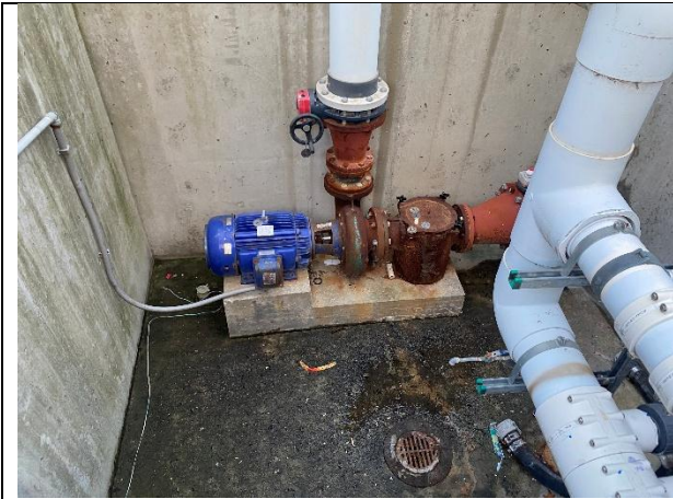
Figure 61 Play feature pump, motor, and strainer
