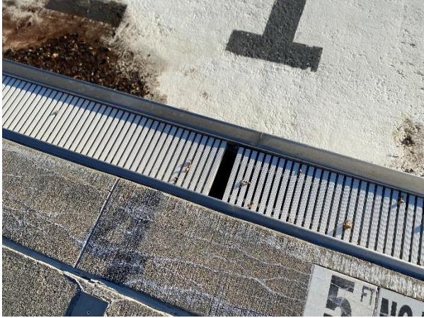
Figure 37 Gap in gutter grating
