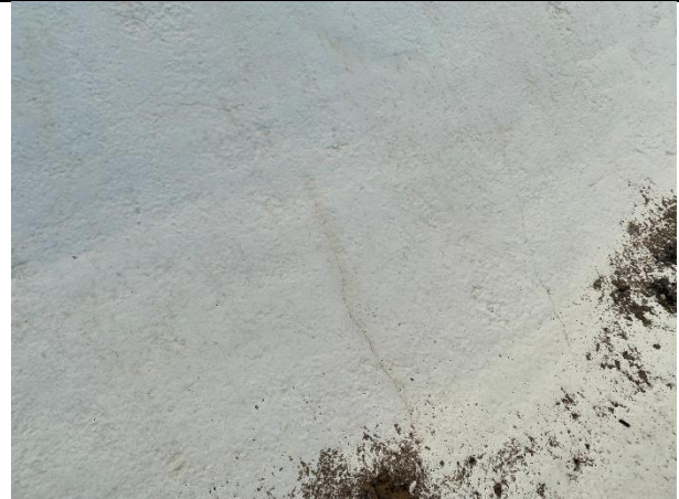
Figure 22 Surface cracking on pool floor
