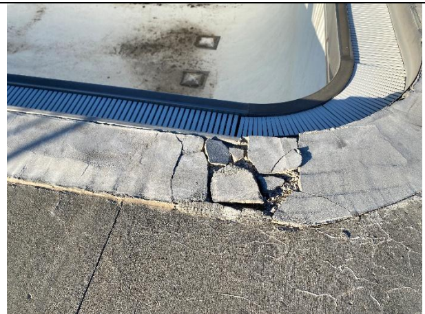
Figure 34 Concrete failure at deck edge to gutter
