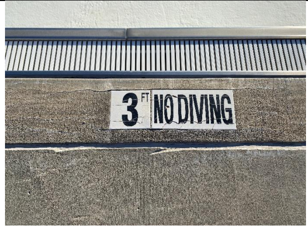
Figure 26 Shrinking caulking and cracking in deck to gutter transition area
