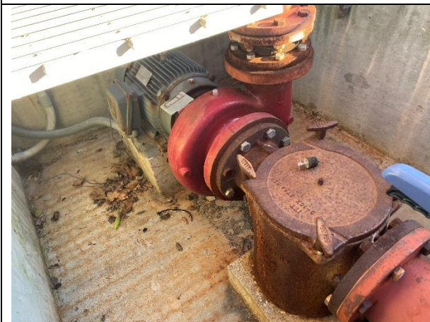
Figure 45 Waterslide pump, motor, strainer
