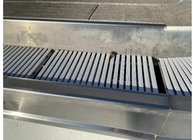
Figure 38 Gaps and bowing in gutter grating
