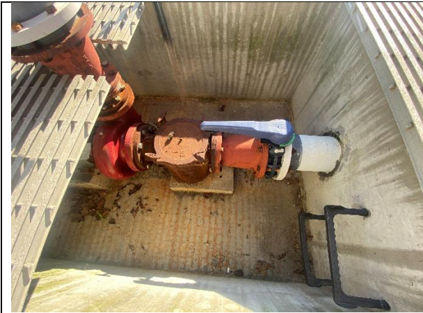
Figure 43 Waterslide pump pit
