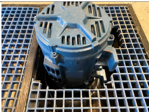
Figure 58 Pool recirculation pump
