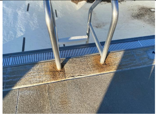
Figure 32 Cracking and corrosion on pool deck by ladder railings
