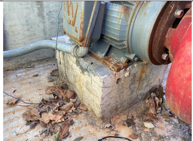
Figure 44 Concrete failing on waterslide pump support base
