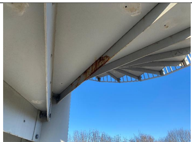
Figure 48 Corrosion on underside of waterslide tower
