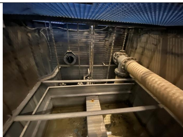
Figure 59 Pool surge pit (previous sand filter)
