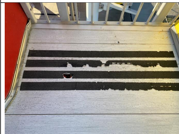
Figure 47 Delaminating non-skid surfacing tape
