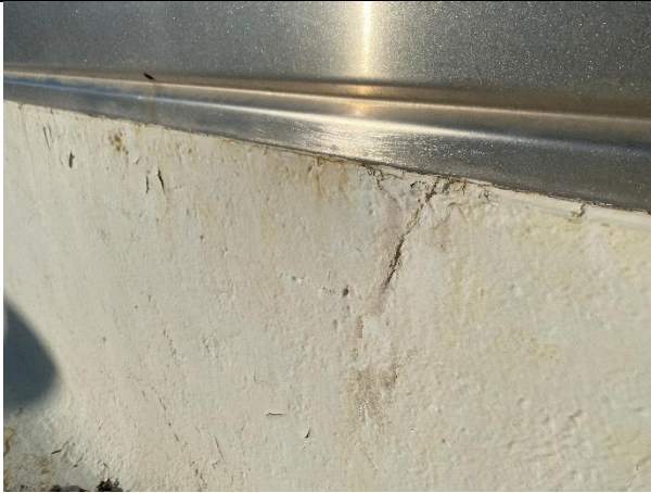
Figure 19 Cracking beneath pool gutter
