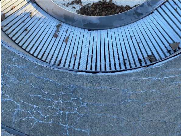
Figure 67 Separation of deck and gutter
