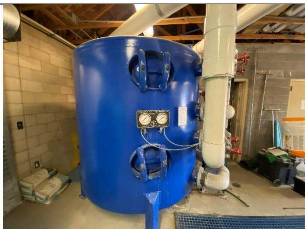
Figure 56 High-rate sand filtration
