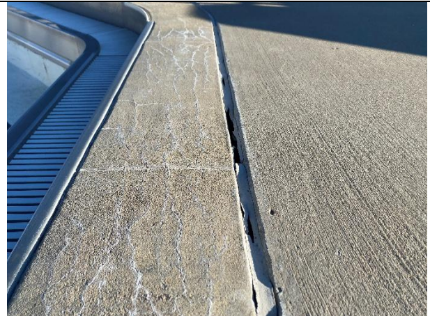
Figure 28 Missing caulking in transition to pool
