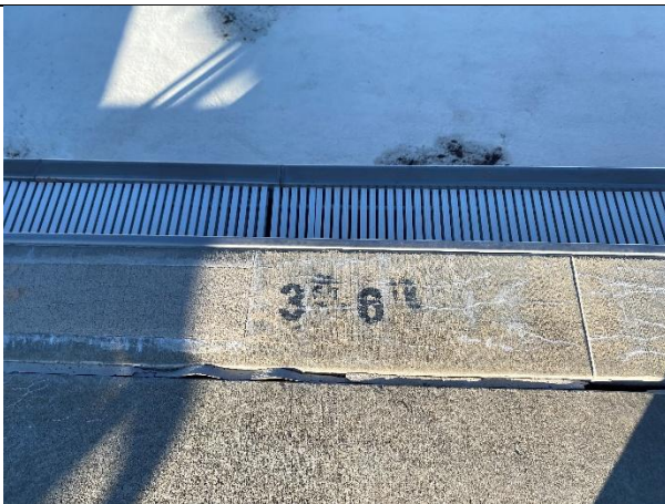
Figure 29 Faded depth marking on deck
