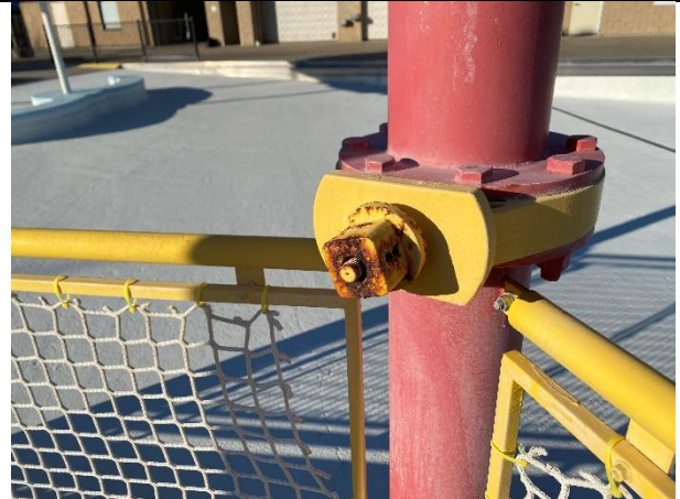
Figure 40 Corrosion on play feature bolt, missing steering wheel feature
