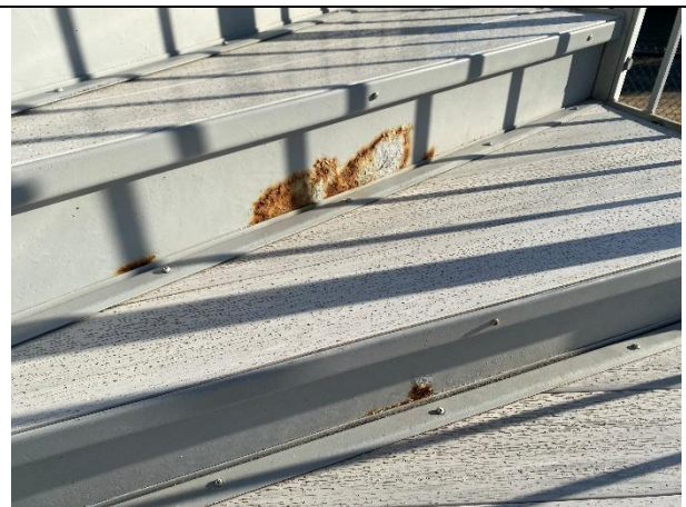
Figure 46 Corrosion on waterslide tower stairs
