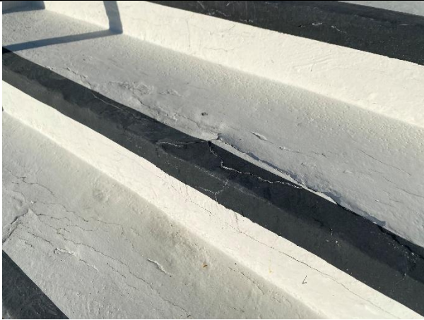
Figure 13 Cracking, heaving and settling in pool stair entry
