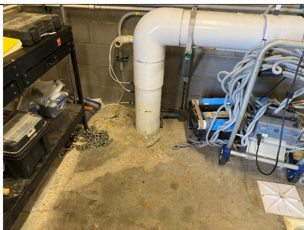
Figure 60 Pool pressure piping
