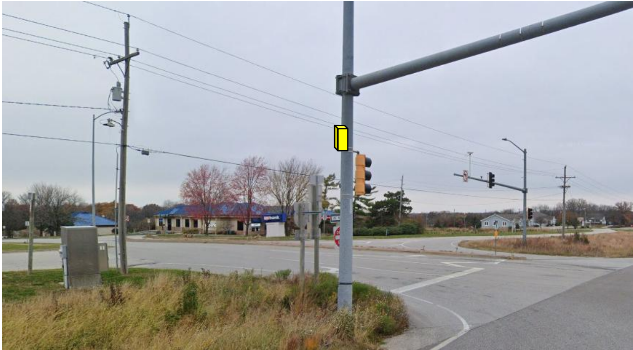
Figure 3: Mounting location of the FCU. Cameras cables will run from the FCU through available conduit to the other structures to connect the cameras.
