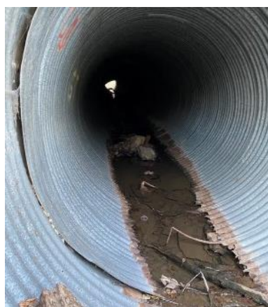
East Barrel: Corroded Invert, Pipe Deformation, Upstream
