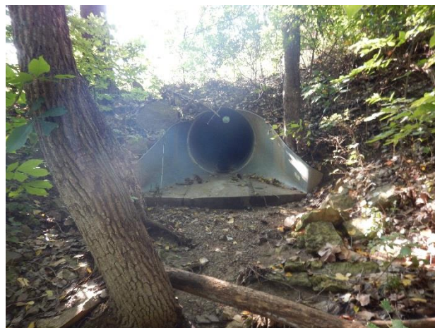
Minimal outlet scour at 60" CMP outfall
