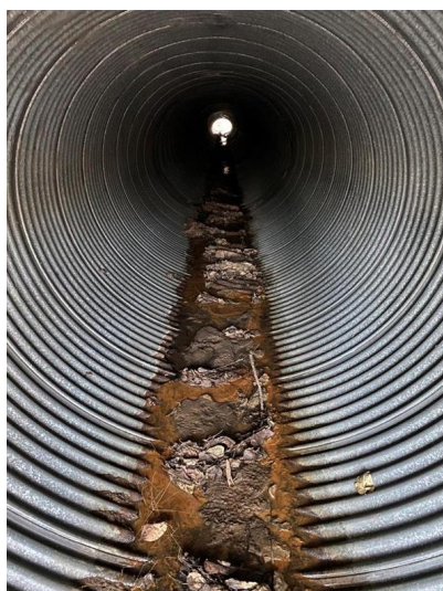
West Barrel: Rusted Invert (Typ.), Upstream
