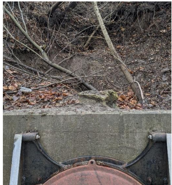
Scour Hole Behind Headwall
