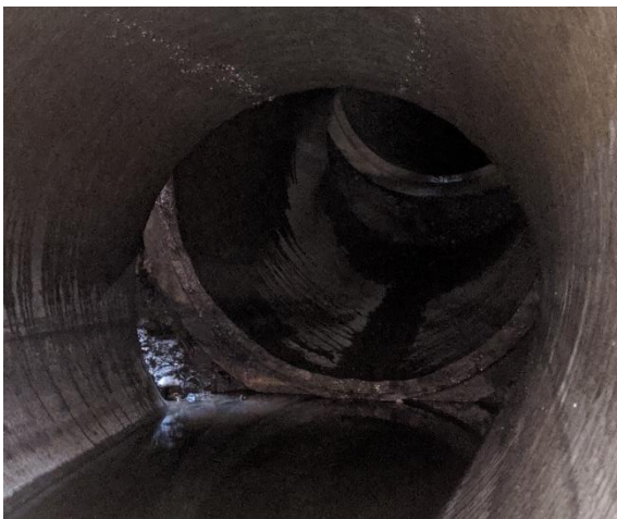
Internal Joint Separation of 48" RCP
