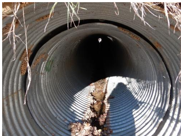
Corroded Invert and Joint Separation (Upstream End)
