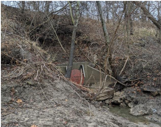
Tilted Headwall & Scour Hole Behind Headwall
