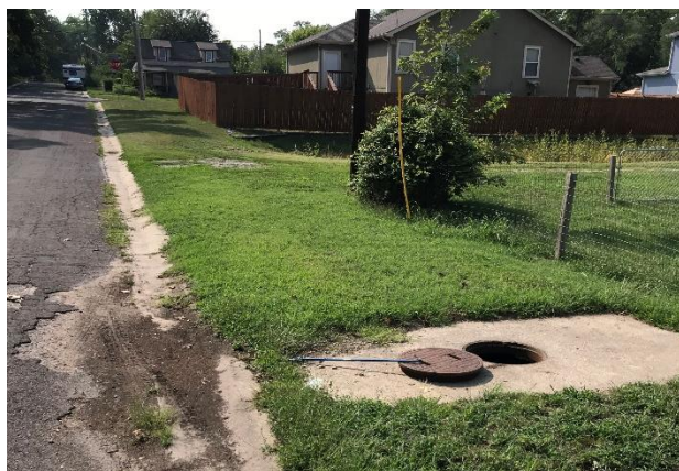
Existing Murphy Ave mid-block junction box near 300 Cornell (Looking west)
