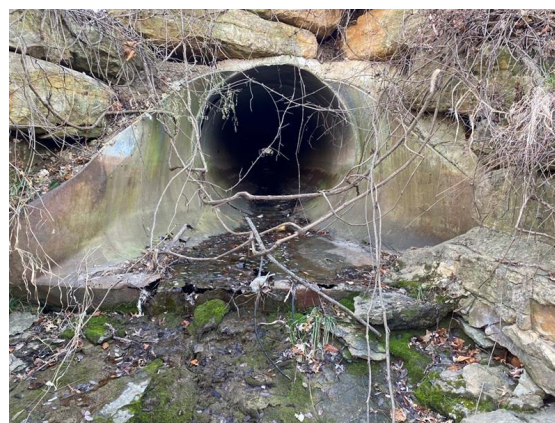
East Barrel: Corrosion of End Section, Downstream
