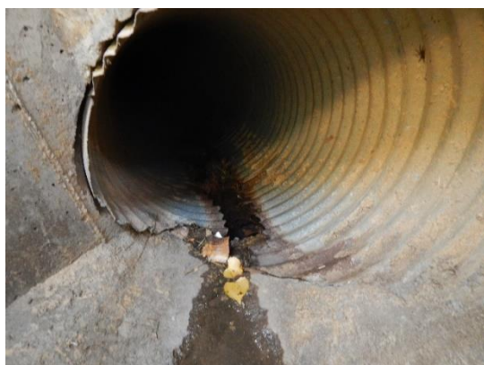
Corroded Metal Pipe at Curb Inlet
