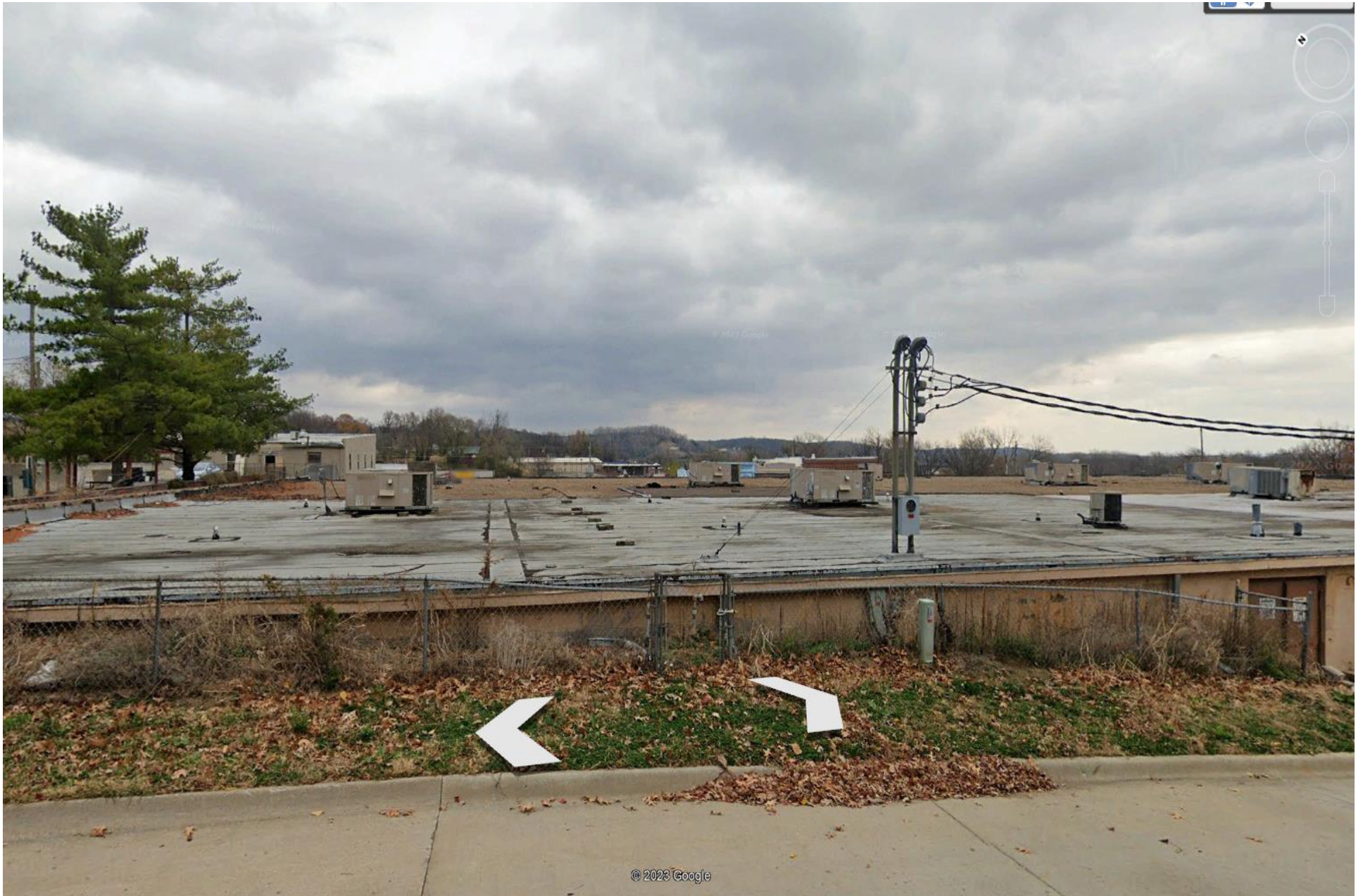
126 Elm previous view, this would look at the upper two floors of the complex
