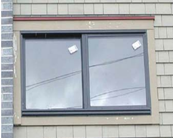
Due to their horizontal proportion, sliding windows are not allowed.
