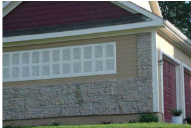
This building has brick that terminates within 4 feet of a corner.
