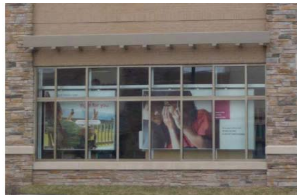
The window opening in the stone wall has no trim; the window frame is at least 2 inches wide.
