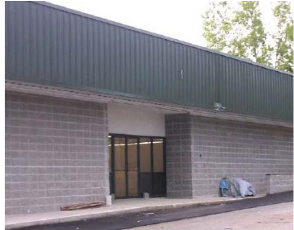
The customer entrance on this building has no detailing.
