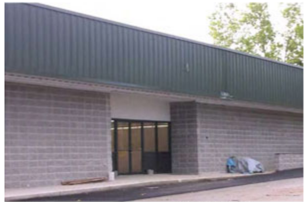
This customer entrance on this building has no detailing.
