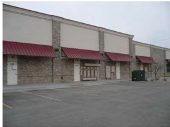
This parapet does not modulate
