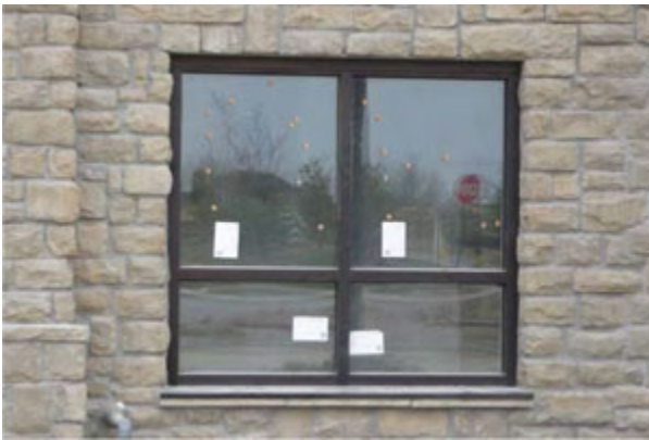
The masonry opening has no lintel, arch, or soldier course.
