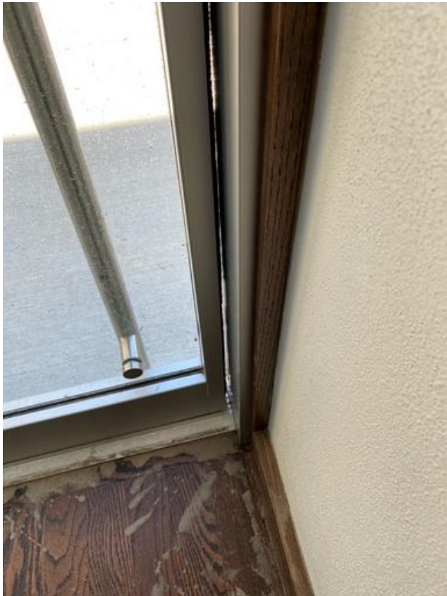
Door Issues 2 SFS Architecture Jun 18, 2021 4:58 PM
