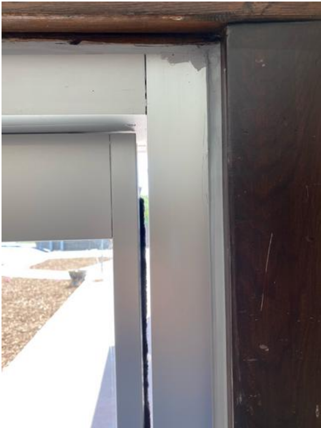
Door Issues 1 SFS Architecture Jun 18, 2021 4:58 PM
