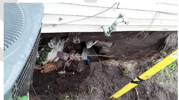
Figure 9. A collapsed foundation from the Labor Day Flood in Manhattan, KS in 2018.
